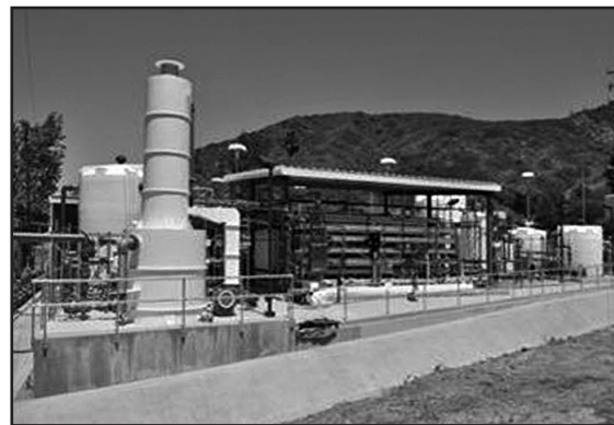
Aliso Creek Water Reclamation Facility
